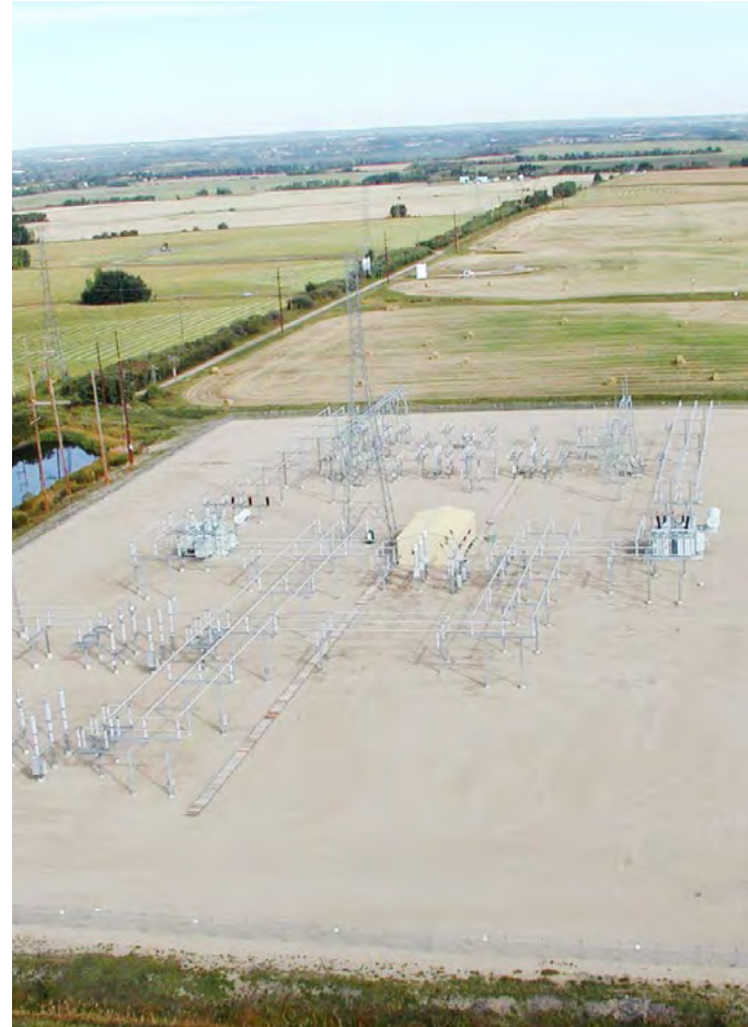
AltaLink's existing Gaetz substation, located east of the City of Red Deer
